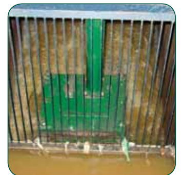
Channel Monster with overflow bar rack.
