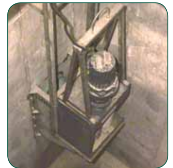
Channel Monster installed in pump station with guide frame.
